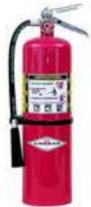
4A rated extinguisher. Sufficient fire protection.
